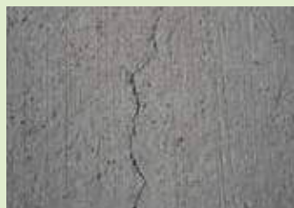
Penetrates into very fine cracks
