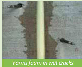
For water bearing cracks
