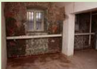
On damp masonry
