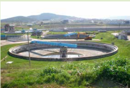
Sewage treatment plant, Istanbul, Turkey
